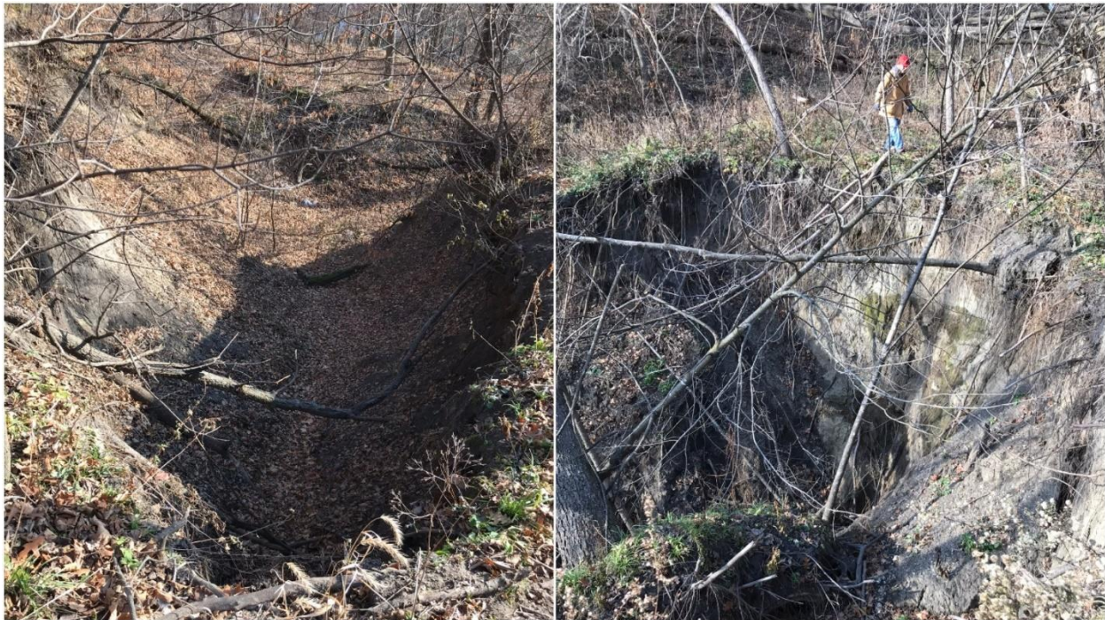
Figure 15. Ravine erosion to the east of the Frederick property.
