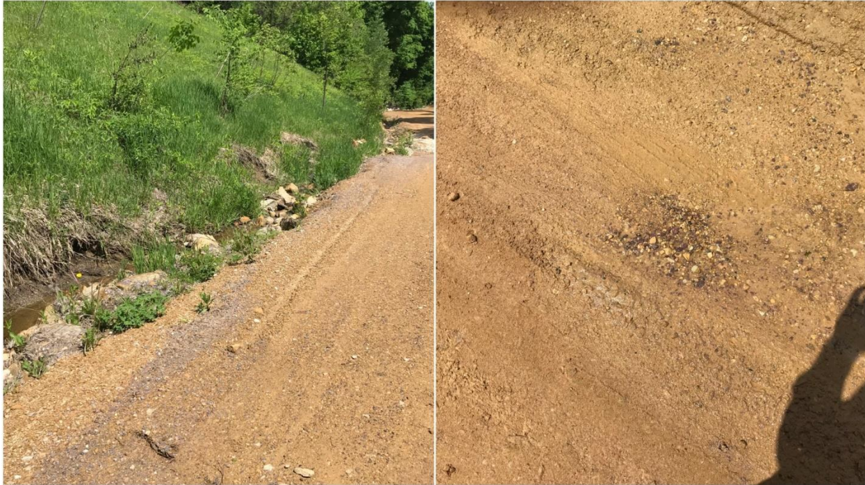
Figure 5. Ditch erosion along the northern side 490th Street (CR28) (left) and groundwater seepage within the roadway (right).
