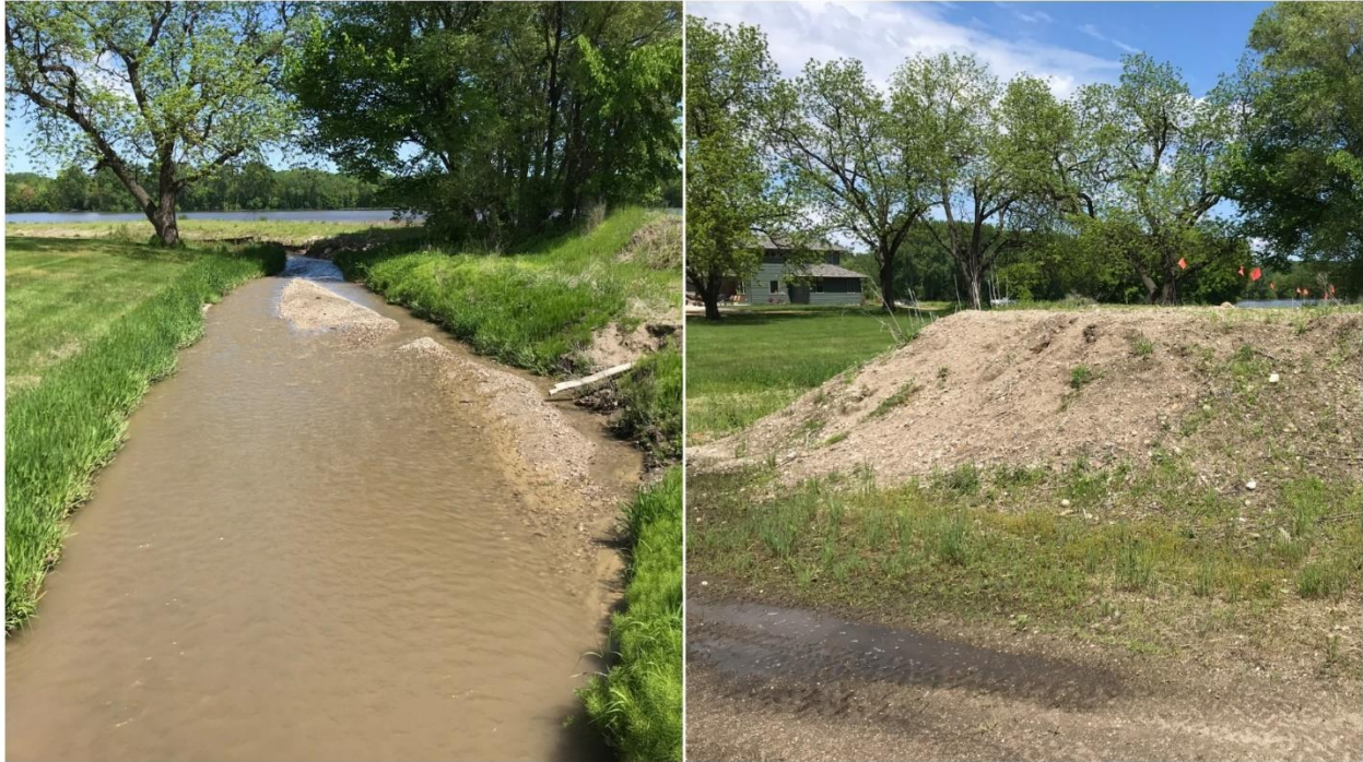
Figure 3. Sediment deposition and pile of removed sediment at the project area outlet near US 169.
